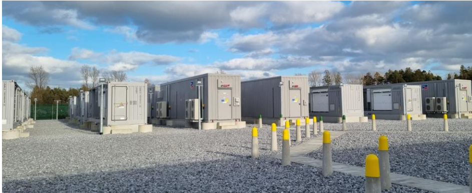
Figure 2.4 Image showing typical arrangement of LDES enclosures
